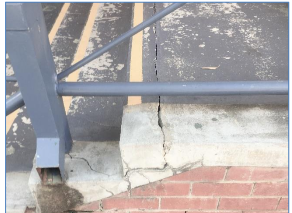
Fig.1 Damaged concrete presenting safety hazards
