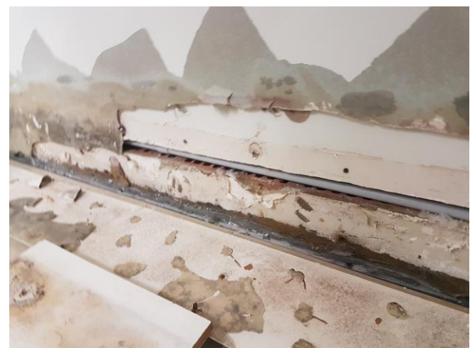
Fig.3 Portion of internal damage caused by the water ingress
