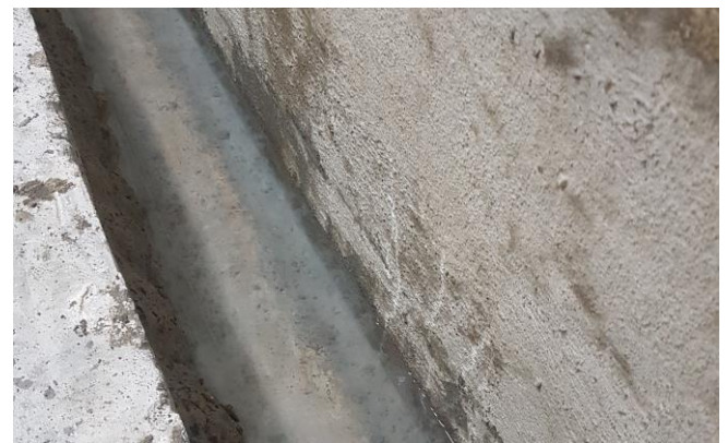
Fig.2 The water ingress at the concrete slab
