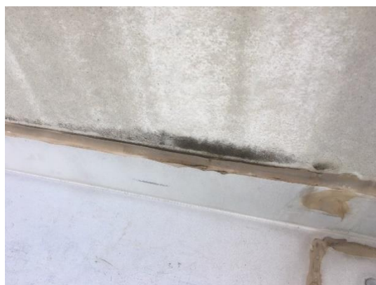
Image 3: Failed joint - window area
