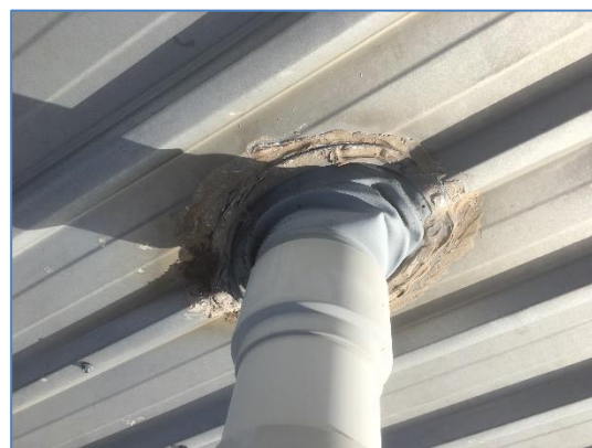
Image 2: Failed seal on roof penetration
