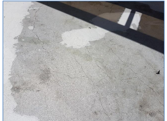
Image 1: Failed waterproofing membrane system
