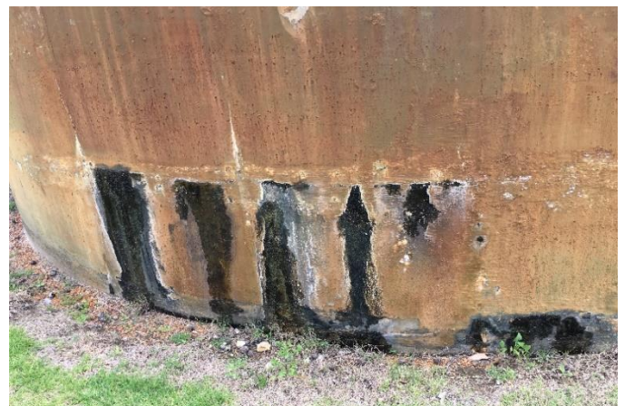
Image 2: Concrete spalling at base of tank
