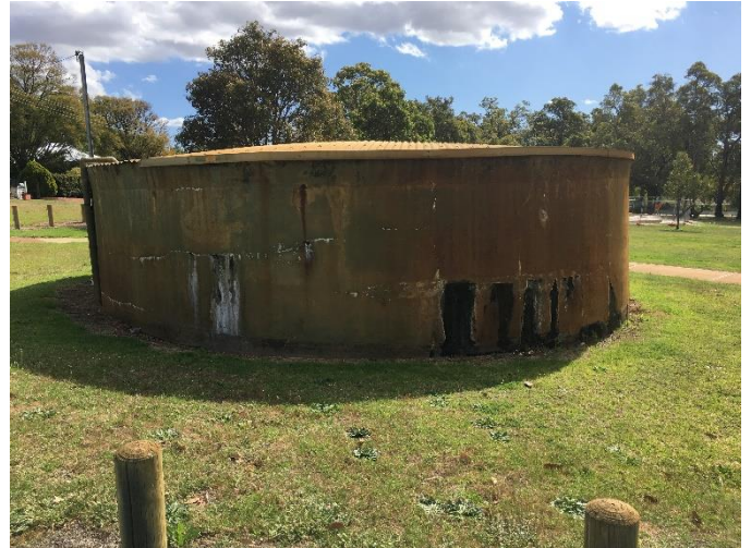
Image 1: Water tank at Collier Park
