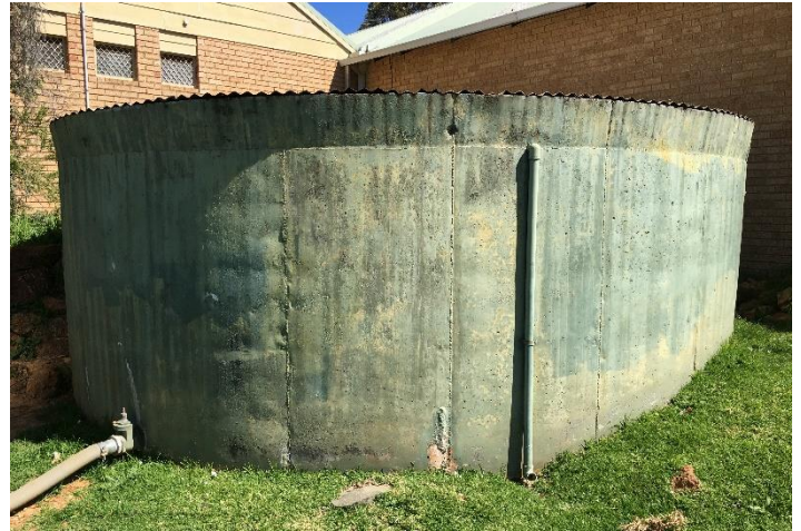
Image 1: Water tank exhibiting various signs of damage
