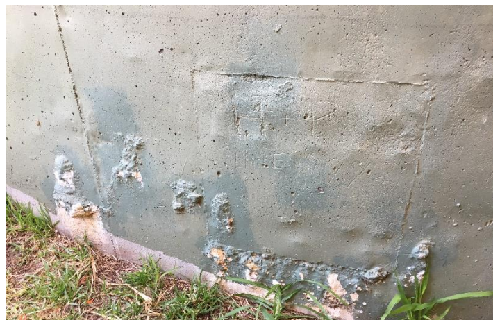
Image 2: One area of damaged concrete
