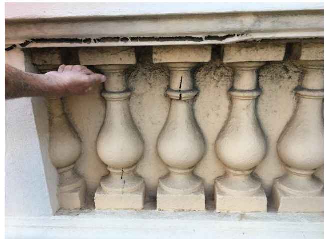
Image 2: Extensive concrete deterioration
