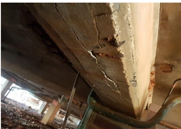
Image 1: Extensive concrete cracking to beams
