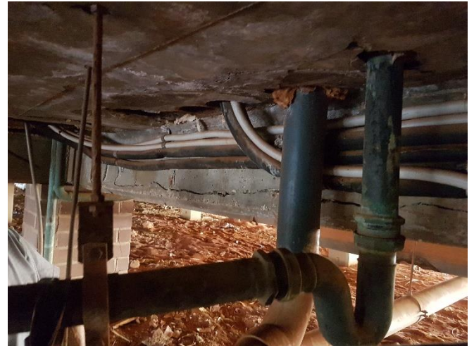
Image 2: Extensive concrete cracking and spalling to underside
