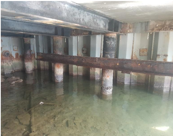
Image 5: Corroded wharf piles
