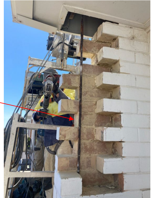
Image 1: Demolition of cracked wall nib bricks exposing corroded roof tie-down
