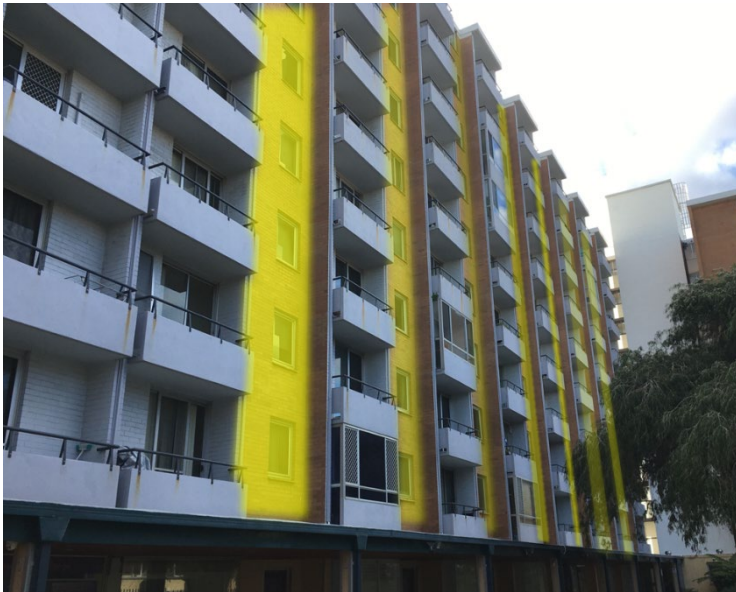
Image 3: Drops (shaded in yellow) to be repointed
