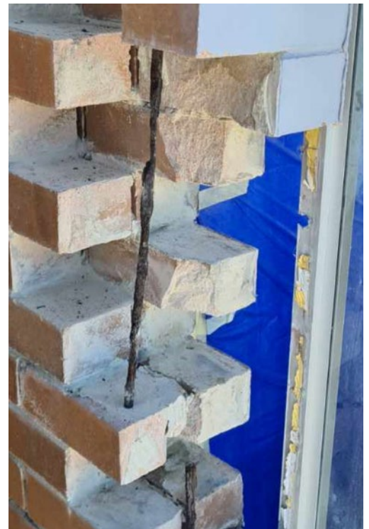
Image 2: Corroded roof tie-down in wall nib
