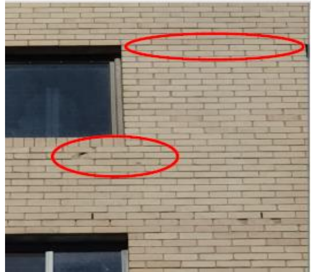
Image 2: Sample of façade areas requiring repointing
